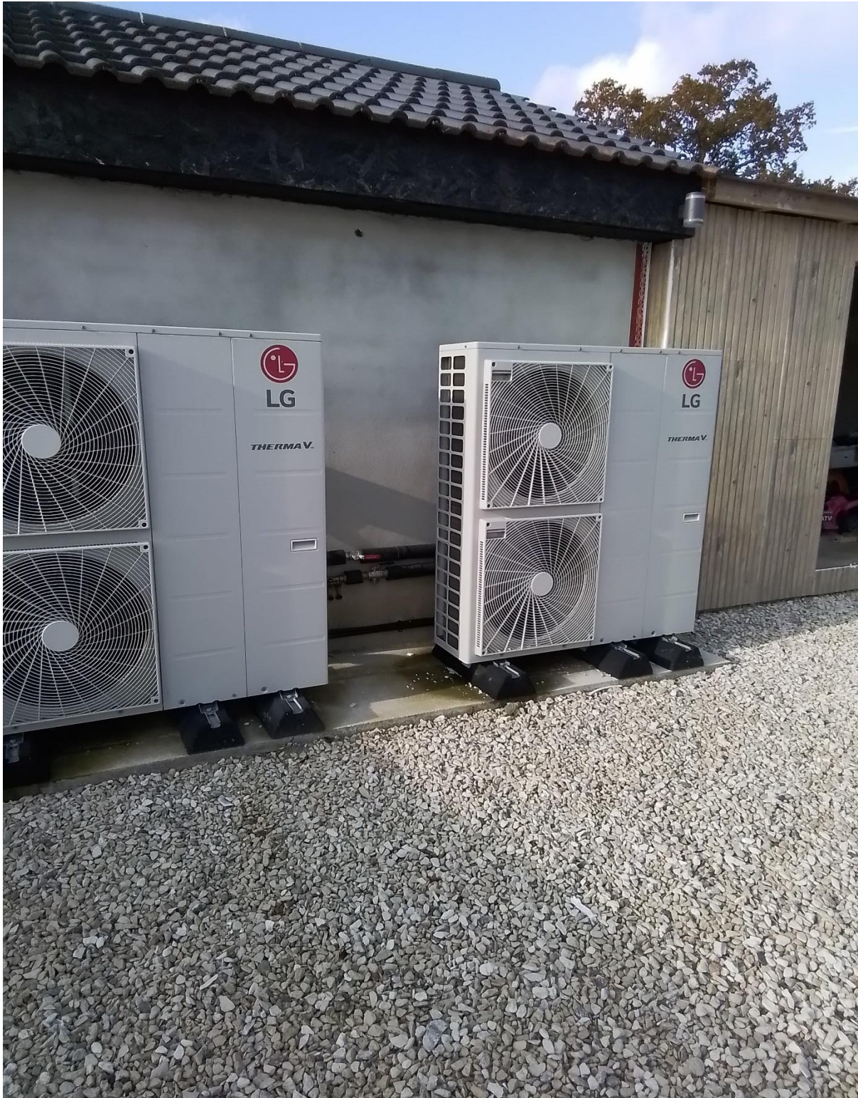
Air con attached to rear of outbuilding Anchor Paddock
